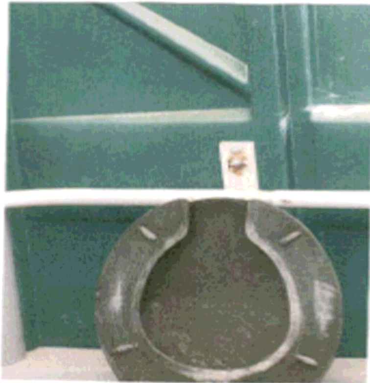
San Jacinto Valley Academy – Porta-Potties at end of sports field. Unsanitary conditions.
